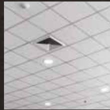
CEILING GRID FALSE CEILING
